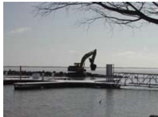
Tradewinds Marina staff race to add height to the levy of Harbor #2—crest of 459.95' made the added rock necessary! (photo courtesy of Jim Mowrey)
